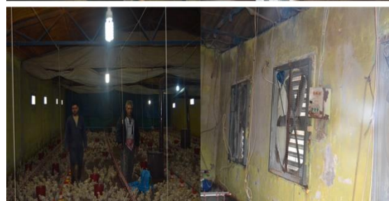
Picture 4. Different windows and ventilation equipments
